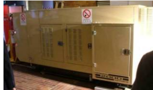
2004 - H2ICE Generator (Generac)
